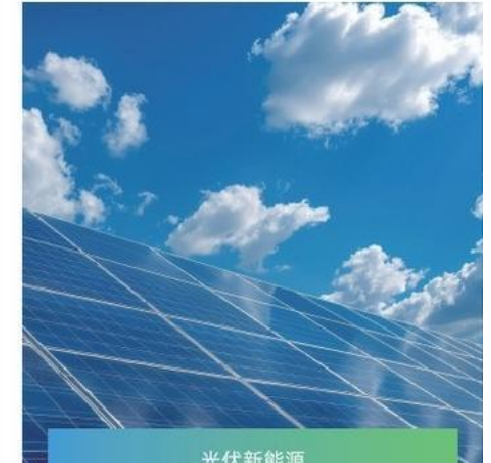
光伏新能源 Photovoltaic new energy
